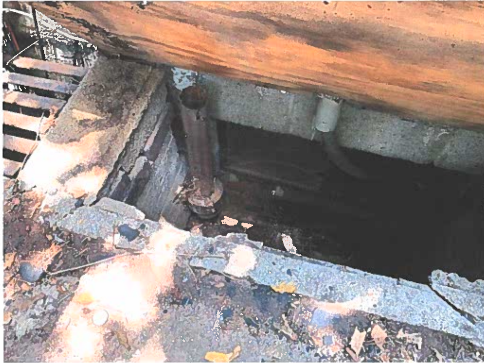
View of past roof leader connection to the sanitary sewer
