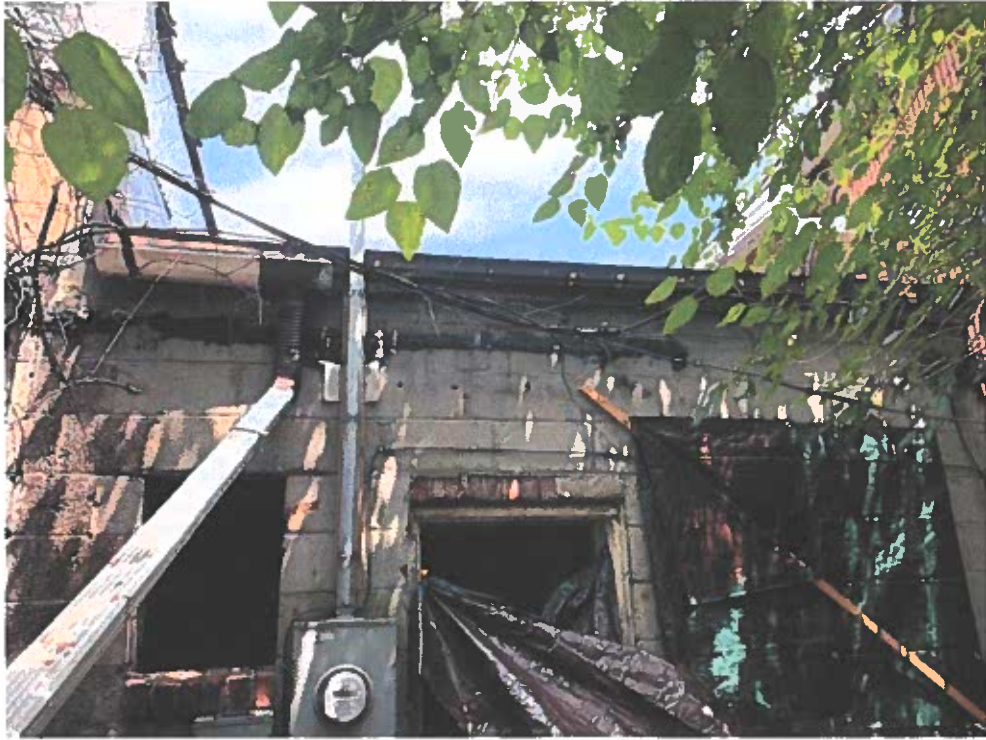
View of roof gutter and roof leader on rear of the building
