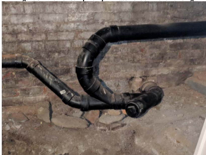
Figure 6 - View of Sewer Lateral Leaving Front Building Through the West Wall Toward North Cedar Street
