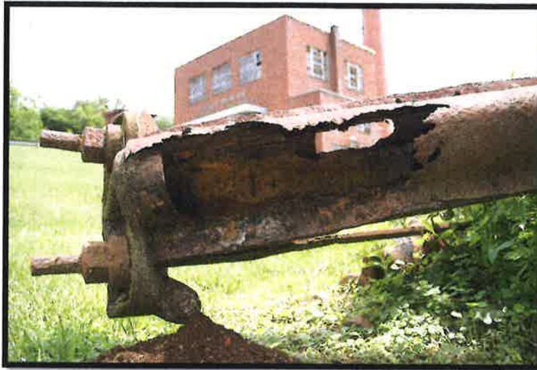
Typical corrosion at abutments L0 top tube and some bottom tube section and plate gone. Arch #4
