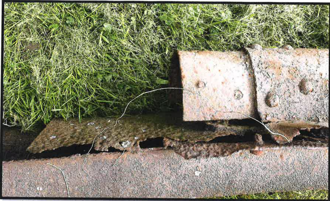
Splice coupling - note coupling riveted to one end of tube in shop and bolted through drilled and tapped hole on adjacent tube section in the field. Note also that plate has completely corroded between the flange of the top and bottom tube sections. Image from arch #6.
