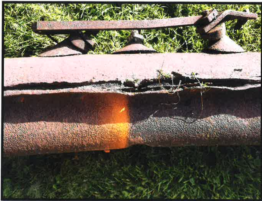
Rust bulge, rivets popped, Arch 1 joint U3, note missing portion of cruciform vertical
