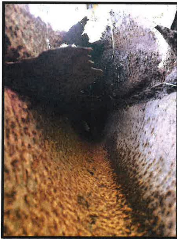
Looking up tube section at L0 for arch #2. Diagonal U1-L1 shown in background
