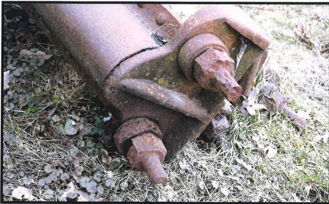
End view of bridge seat and corroded threads from lower tension straps.
