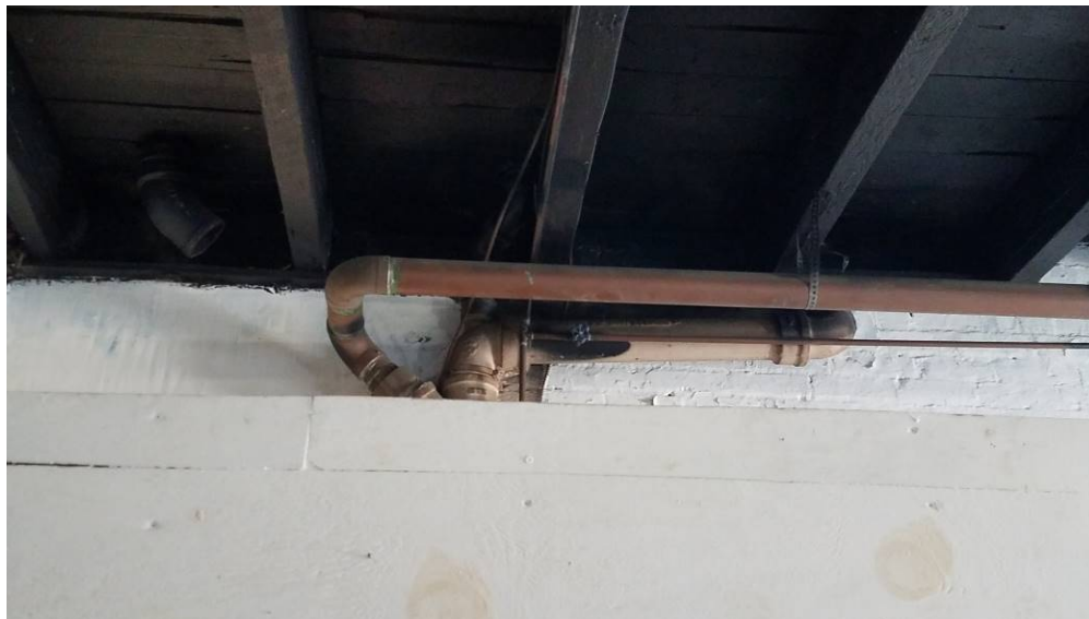
Photo 2: View of plumbing from first floor beneath presumed former second floor bathroom
