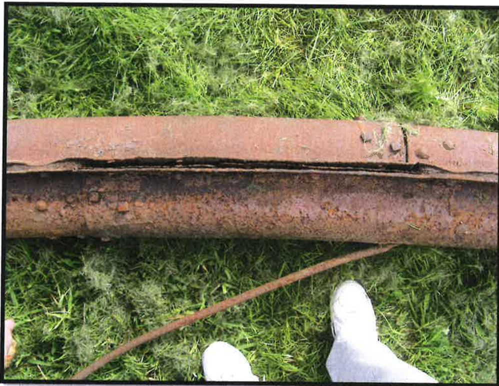
Note existing splice connection on top tube and lower tube members. Some riveted some bolted. Also note rust bulge, rivets popped and probable plate corrosion. Arch #1
