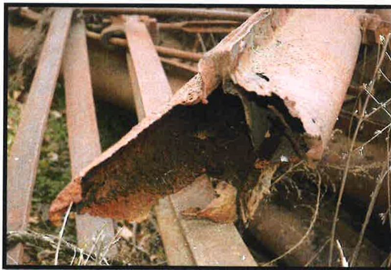
Corrosion showing top and bottom semi-ellipse and middle plate gone
