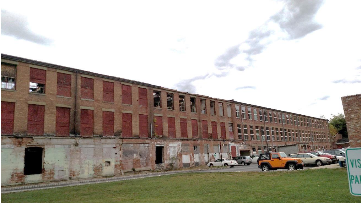
Photo 5: View to the north of Building 16 which is located adjacent to Building 10. Building 10 is currently residential apartments.
